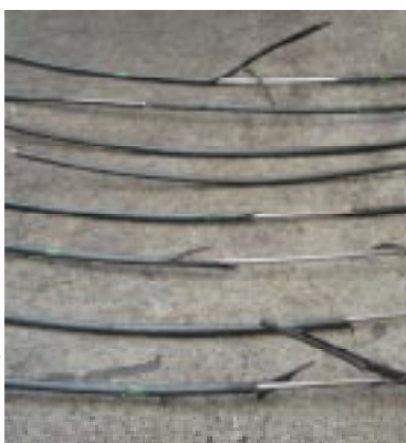
Damaged encapsulated tubewire
